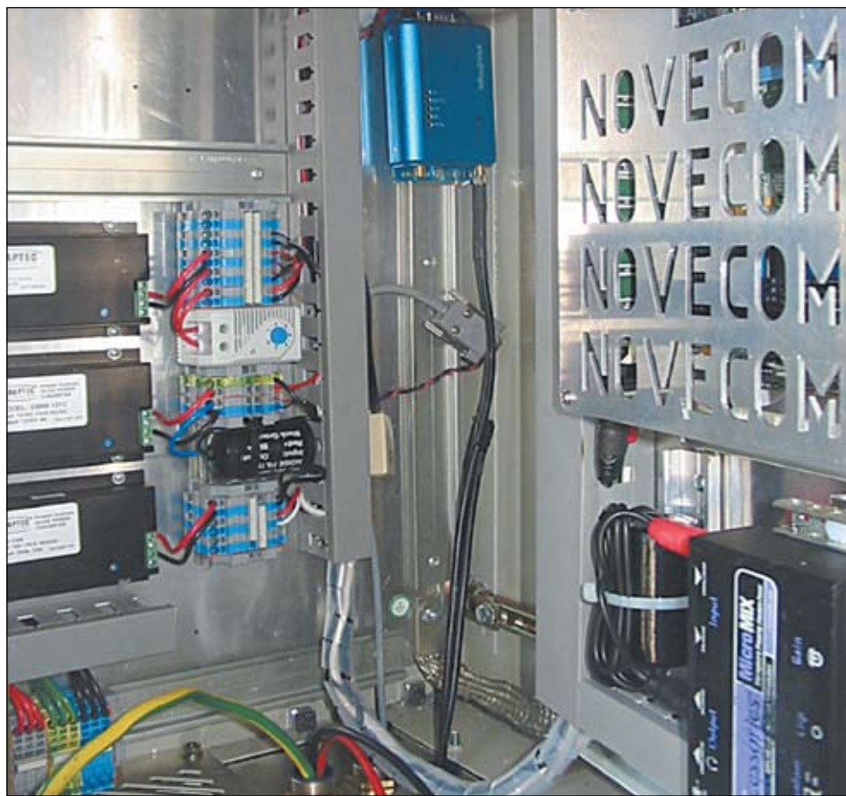
ModMax modem inside a Novecom Sentinex Noise Unit. Maxon's ModMax provides the Sentinex with effective wireless communications
